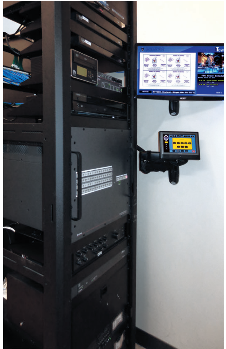
AMS technicians use Extron GlobalViewer Enterprise to independently monitor and route content among the AV systems located across campus.
