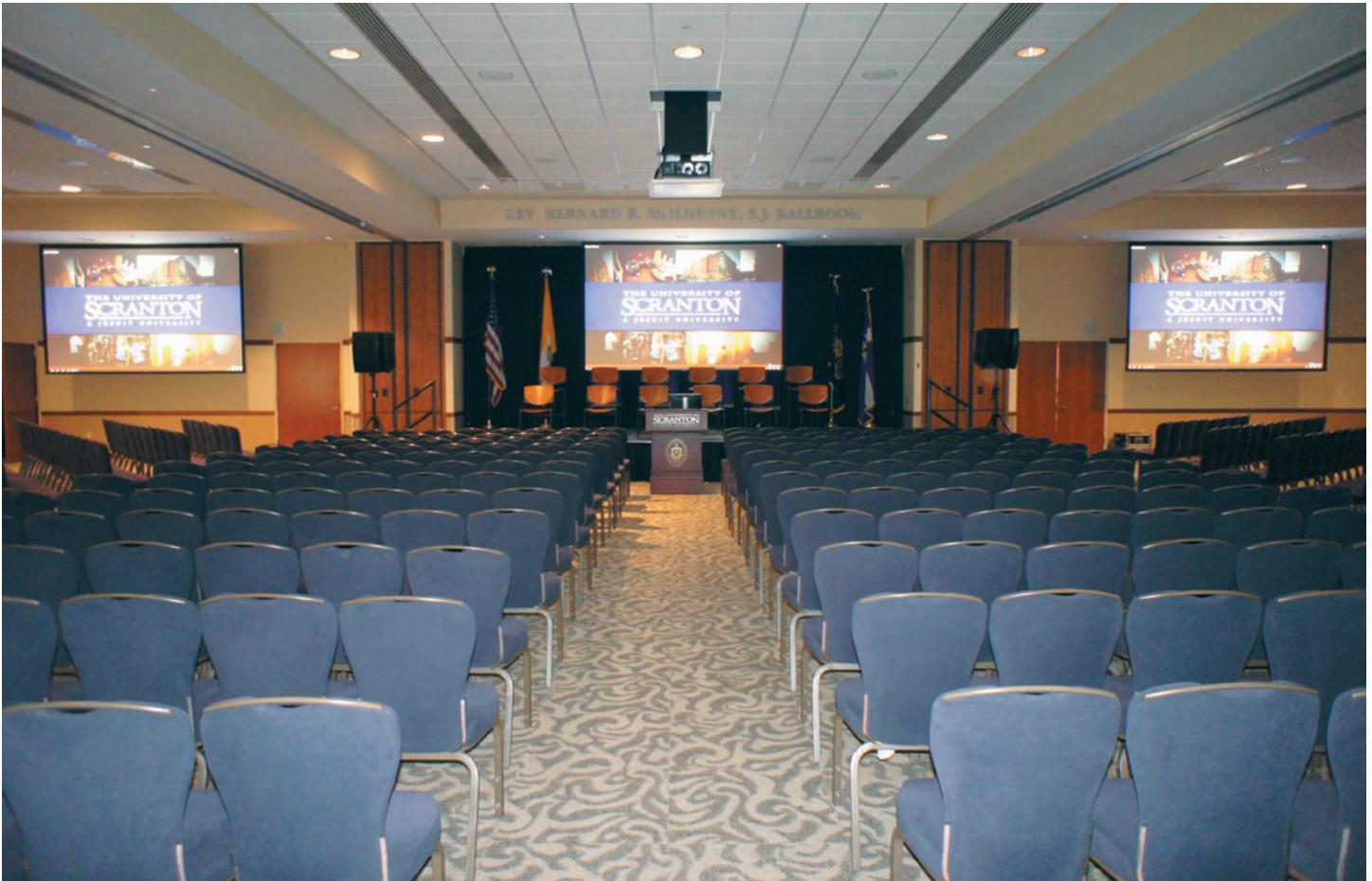
The McIlhenny Ballroom can be divided into two or three meeting spaces, each with independent media control through a shared XTP CrossPoint matrix switcher.
