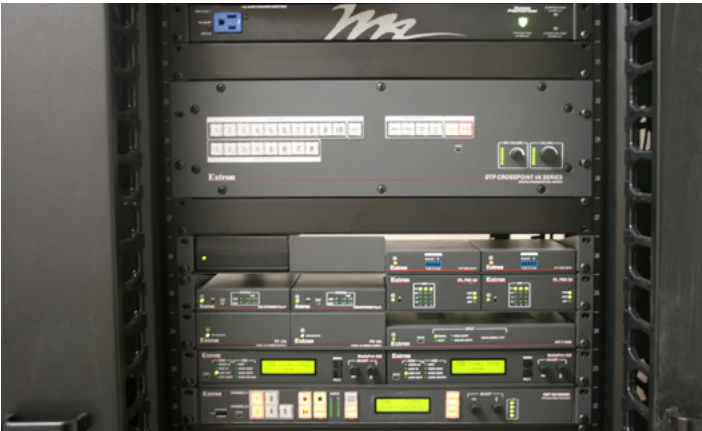
An Extron DTP CrossPoint 4K matrix switcher installed in the lectern provides AV switching, signal extension, audio amplification, and system control processing.
