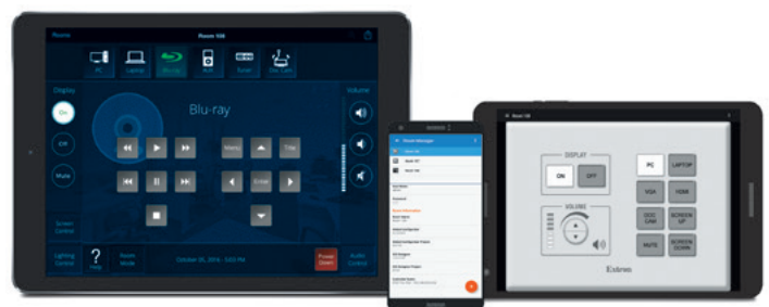
The AV system is controlled using the Extron TouchLink Pro touchpanel mounted near the main entry or from a mobile device that includes the Extron Control app.
