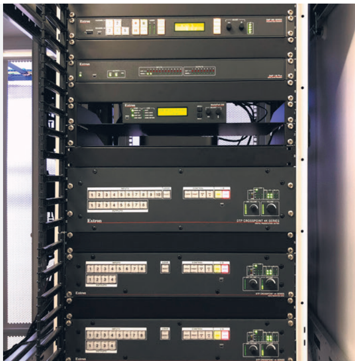
SMP 351 streaming media processor (top of rack) allows classroom training sessions to be broadcast to remote locations or recorded for video on demand. DTP CrossPoint 4K presentation matrix switchers (middle of rack) provide 4K switching and scaling, as well as integrated control processing and audio amplification.
