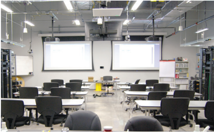
AV in training classrooms allows students to view table-top demonstrations on the projection screens without leaving their seats. Ceiling-mounted flat panel display faces instructor. (Photo Courtesy of BICSI)
