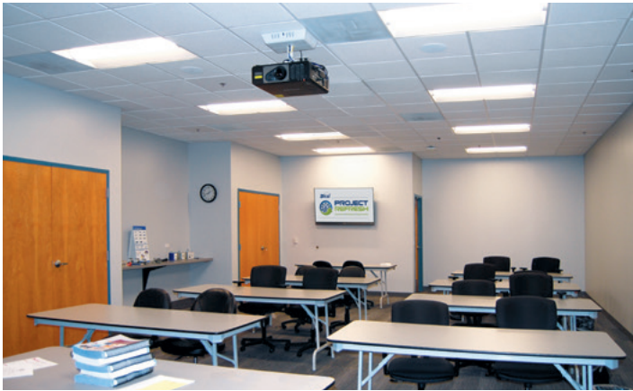
PoleVault Digital System in the design classroom provides AV switching, control, and stereo audio amplification for presentation of multimedia instructional material. (Photo Courtesy of BICSI).
