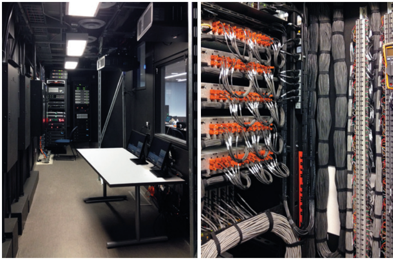
LEFT: Placing racks in a facility's central control room helps reduce noise in DVP-enabled spaces and provides a cool environment for the equipment. RIGHT: Cabling is neatly bundled and properly labeled according to best practices.
