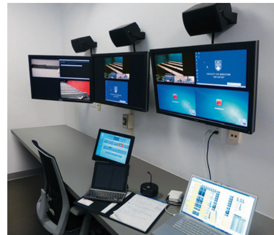
The central control room at an active site operates the TEL system for a facility that lacks the space for a local control room.
